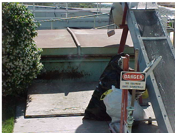
Holding Bin for solids
