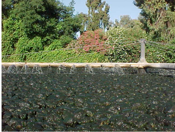
Arms eroding, pinhole. No replacement parts available due to age of equipment.
